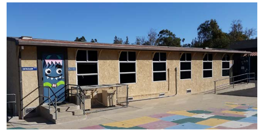
Photo 5 One must use stairs to access the Maker Space Classroom. Access to adjacent general classroom is by way of ramp.
